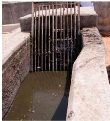
Fig 2: A typical manual screen channel in the septage plant. (Source: Linda Strande)
