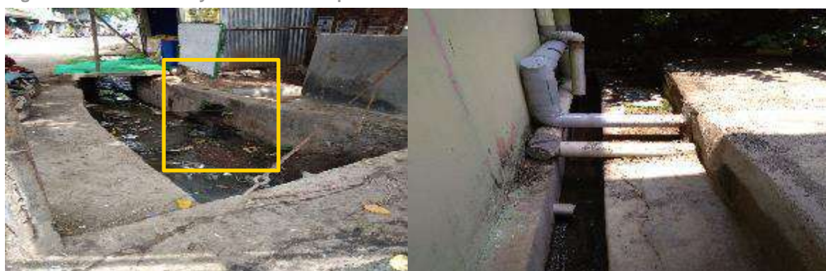
Figure 4-3:-Toilet directly connected to Open and closed drains
