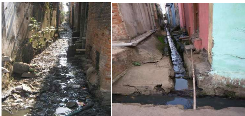
Figure: 4-3 – Households directly connected to open drains
