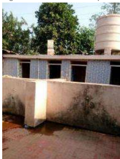
Figure 4-6: -New CTs set-up under Project Samman
