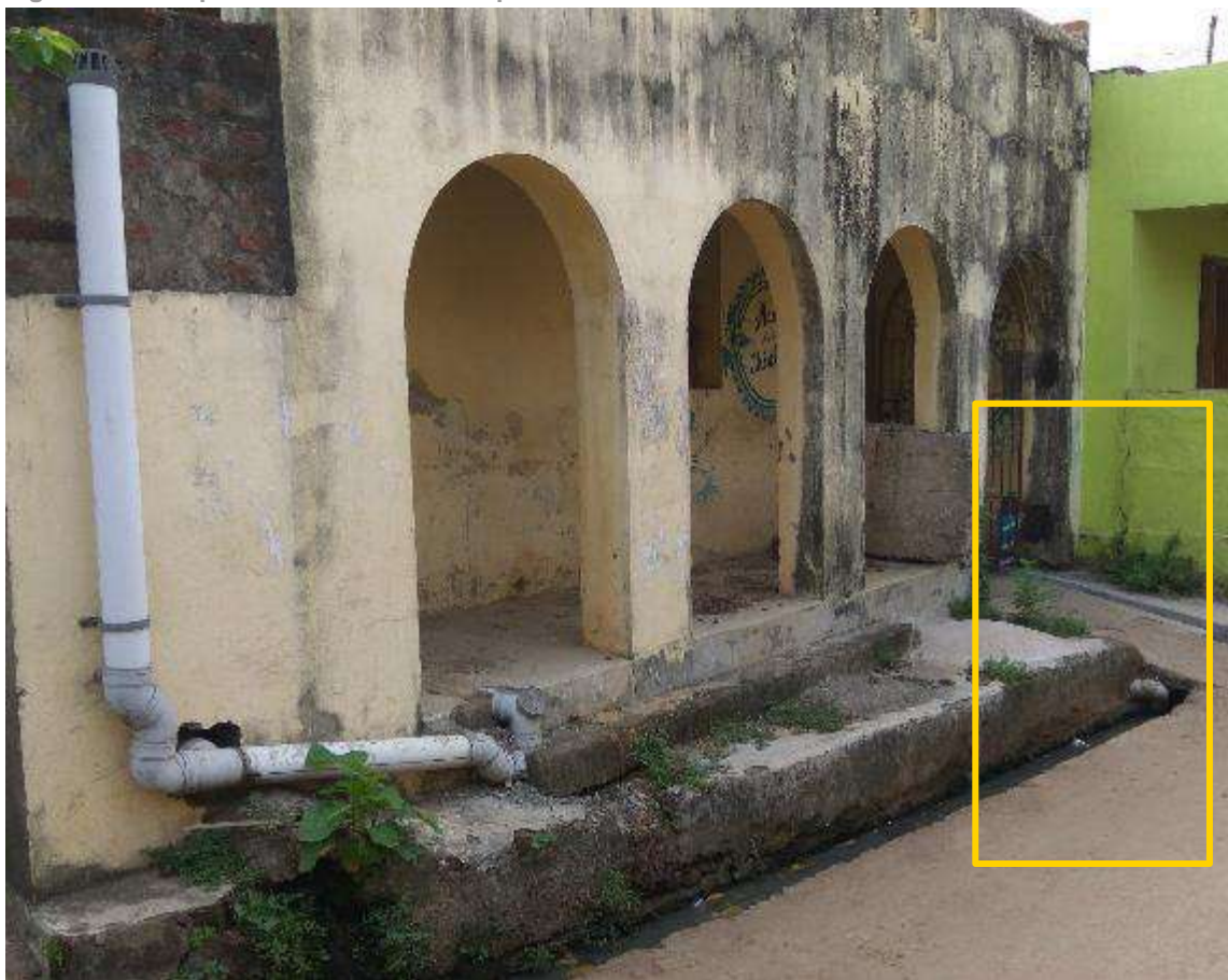
Figure 4-3 : - Septic tank connected to open drain
