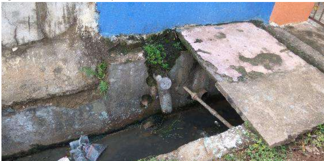
Figure 4-4 :- Toilet connected to open drain
