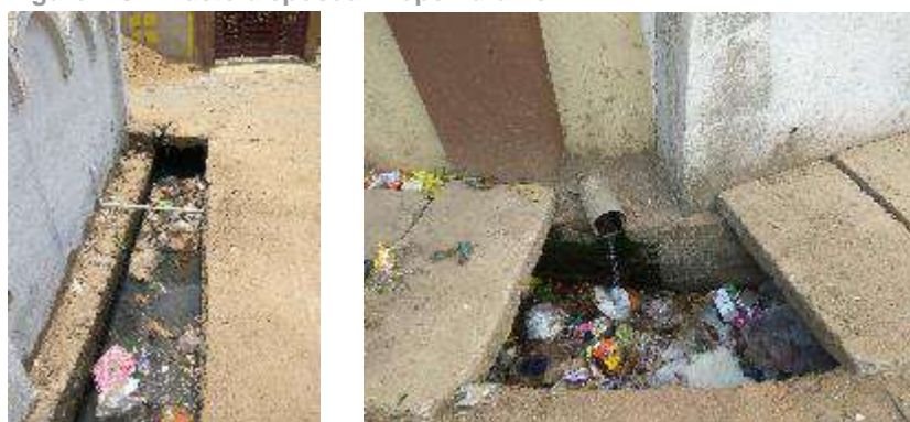
Figure 2-8: -Waste disposed in open drains
