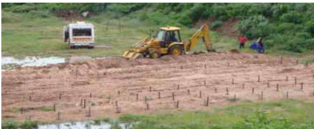
Figure 4-15: - Example of typical deep row entrenchment site
